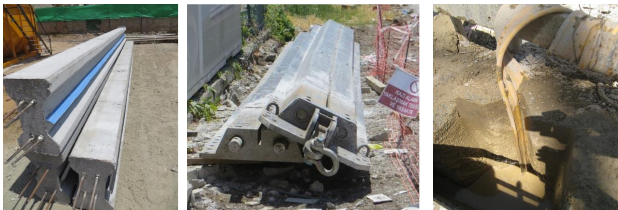
Figure 14. Prefabricated Concrete Elements (left), Steel forms for CWS system (middle), Exposed CWS joint (right)
