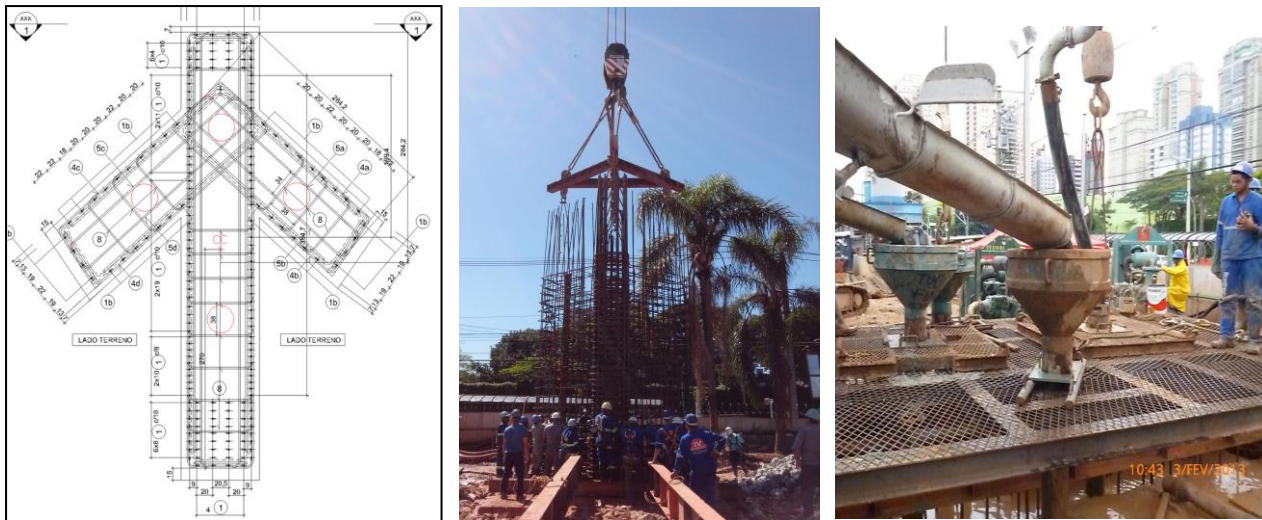
Figure 25. Cage layout with tremie pipe gaps (left), Installation of cage into arrow (middle), Concreting arrow (right)
